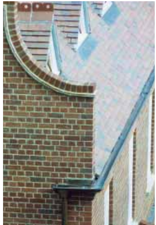
Copper gutters, downpipes, flashings and weatherings at Linacre College, Oxford (BREEAM Gold Medal). Architect: ECD Partnership. Roofing Contractor: Cotswold Metal Roofing.
